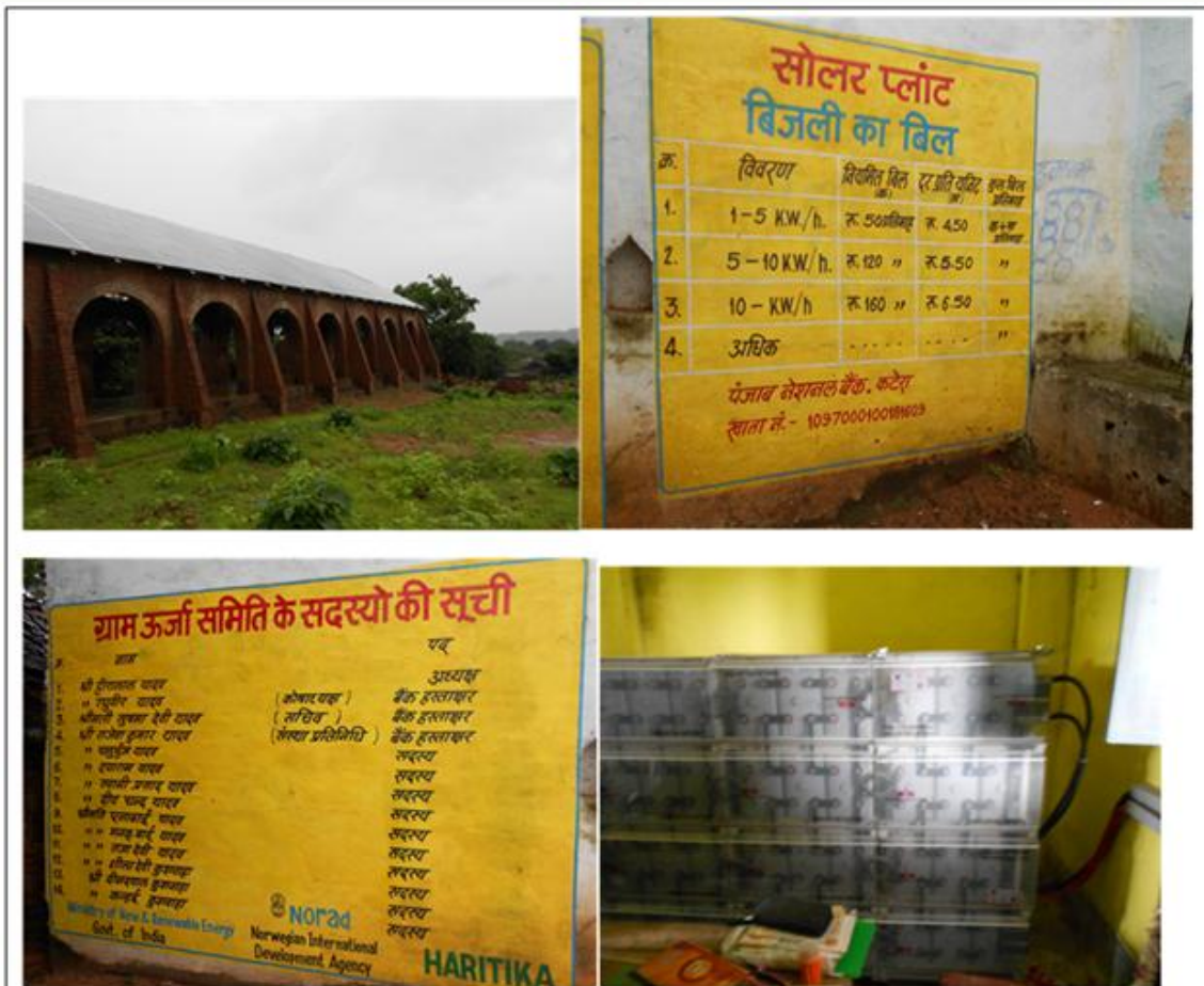
Photos (Clockwise from top left): 25kW Solar PV Plant; Billing scenario of solar electricity; Details of the Village Energy Committee formed for management of the plant; Battery Bank of the plant and leakage in the walls of the equipment room
